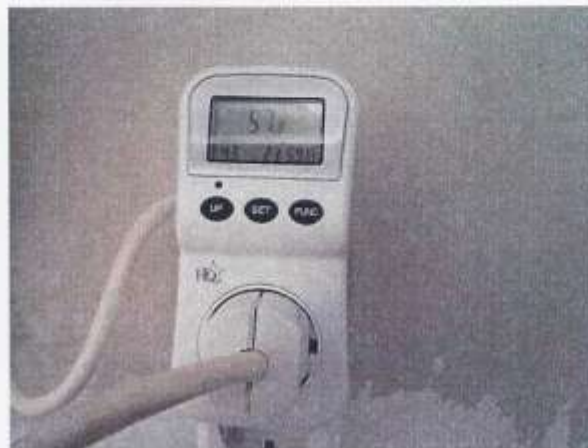
Figure 40. Energy meter in Test Room 2.
