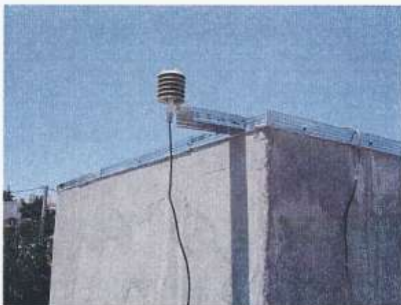
Figure 11. Ambient temperature sensor.
